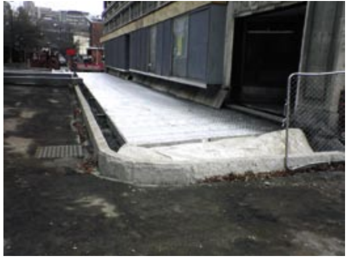
Further sidewalk progress. These sidewalks all have underground vaults so the subframing was all replaced and then waterproofed. Radiant heating was also installed to maintain the walk in snow and ice conditions.
