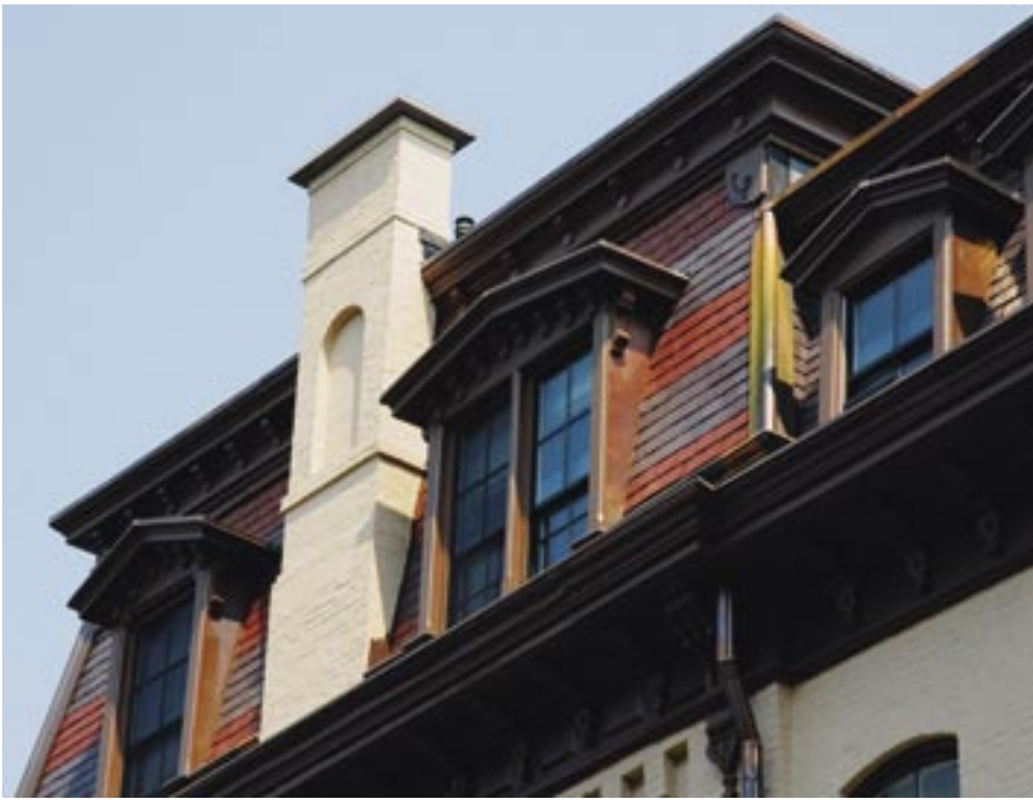
The slate work, completed in phase two, and masonry reconstruction, completed in phase one, are all new and historically correct, including the rebuilt chimneys.
